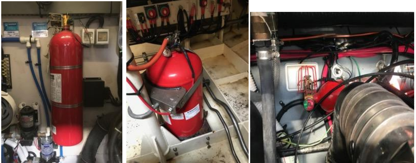
Some examples of fire suppression systems on marine vessels.
